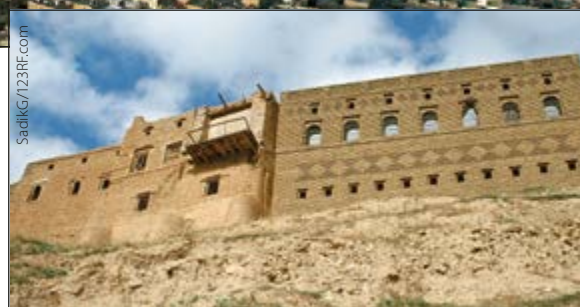
The walls of the houses which form the walls of the Citadel are highly decorated.
