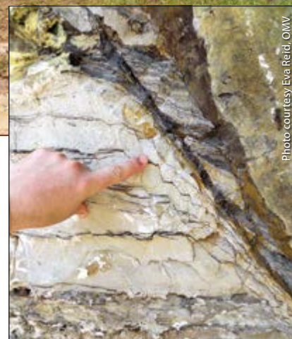
Close-up of the central portion of the fault. Note the complexity when viewed at this scale, including shale smear (continuous in this photograph), internal blocks bounded by two main slip planes and damage to the footwall (left).
