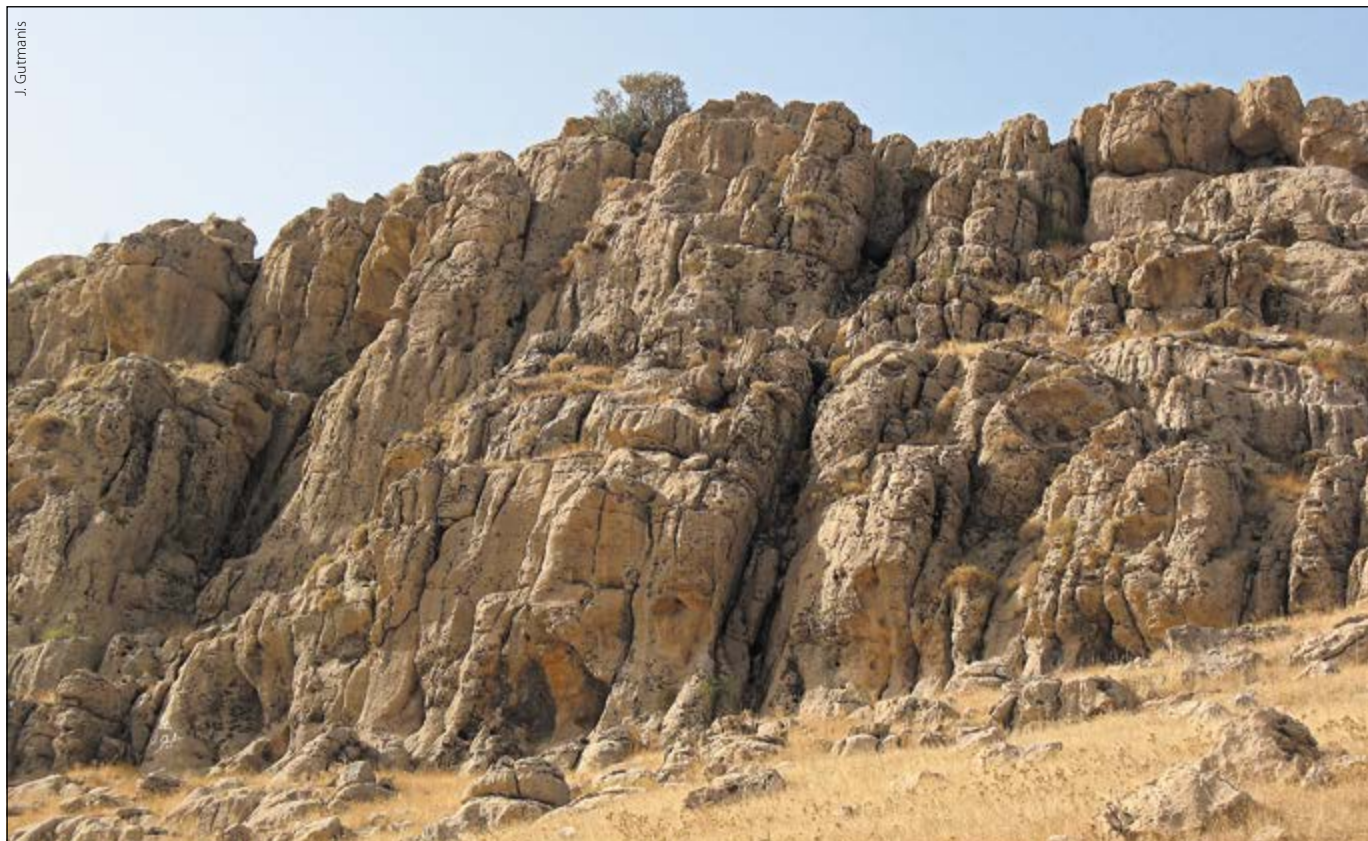
Stratabound fractures and fracture corridors in the Sinjar Formation (Lower Eocene) near Sulaymaniyah.
