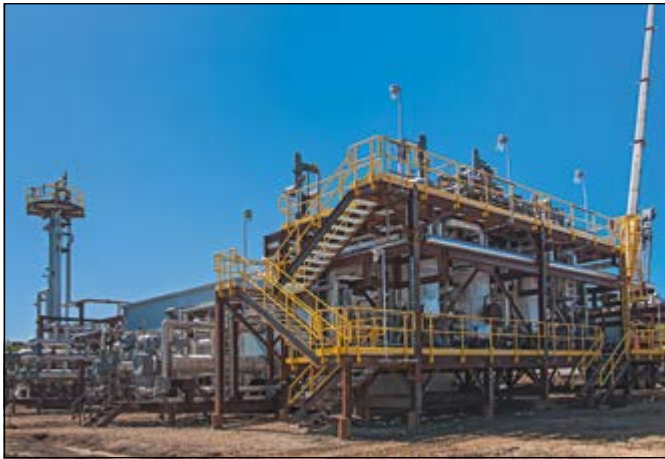
Close-up of NSolv's pilot project in the Canadian oil sands.
