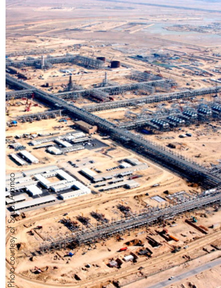
View of the Qatif Central Producing Plants during its construction in the early 2000s. Completed in 2004, these facilities, according to Saudi Aramco, produce 800,000 barrels per day from rejuvenation of the onshore Qatif field (first produced in 1951) and the offshore Ab Safah field (first produced in 1966).
