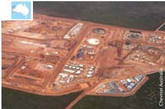
Aerial view of the Gorgon LNG plant site being built on Barrow Island, 56km off the north-west coast of Western Australia
