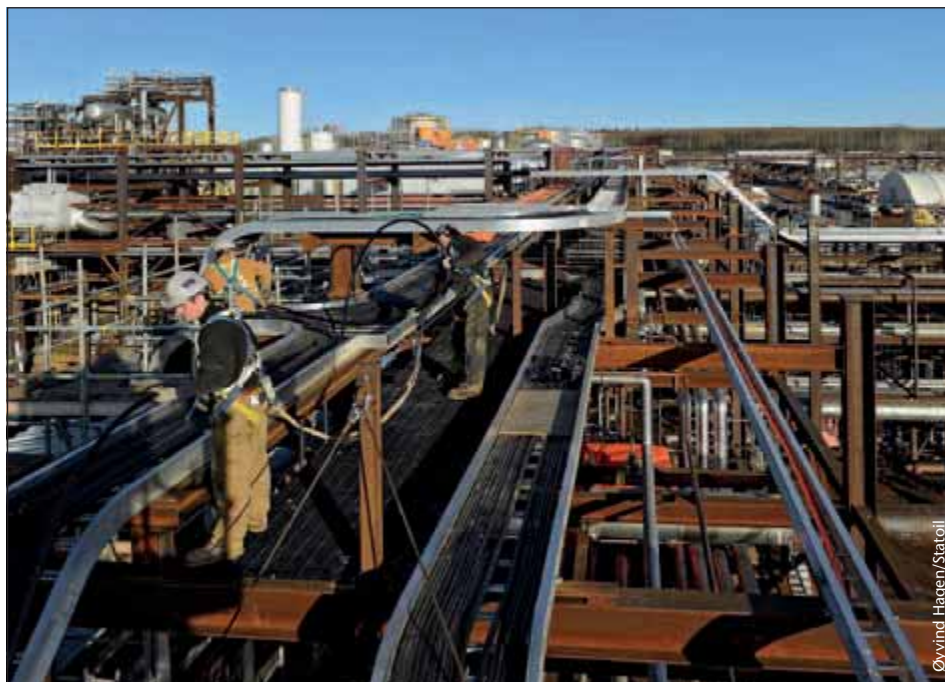
The Leismer heavy oil facility uses steam-assisted gravity drainage to extract oil from heavy oil sands in the Athabasca region of Alberta
