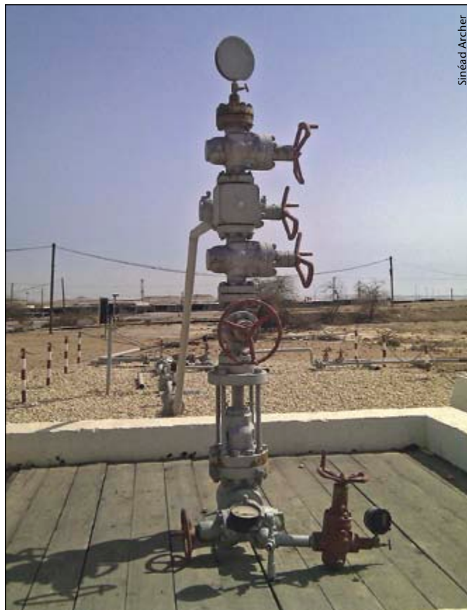
Well Number 1, drilled in 1932 and the first discovery in the Arabian Gulf
