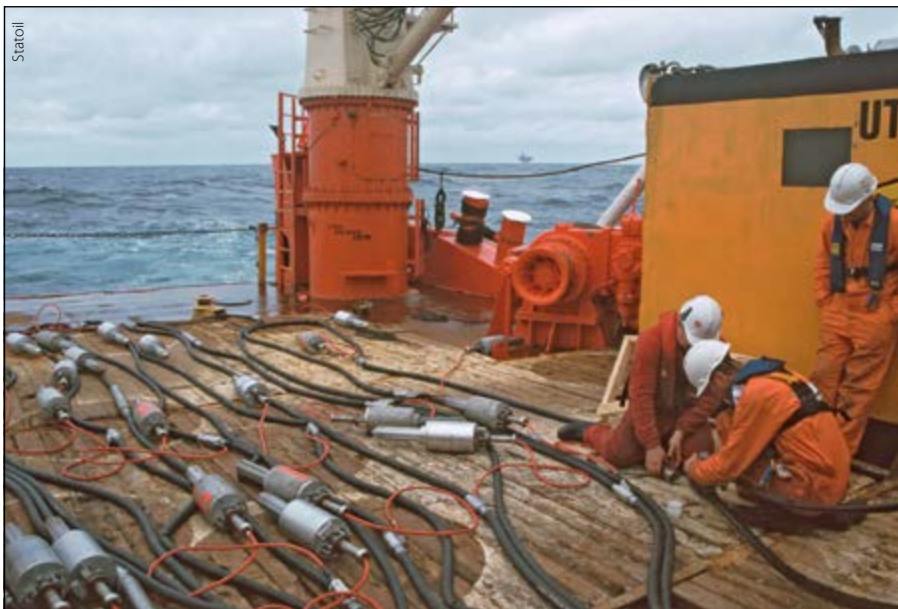
SUMIC nodes ready for deployment with the help of ROVs over the Tommeliten field in 1993.
