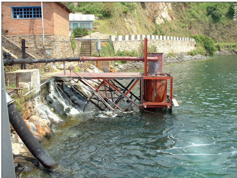
Figure 3: A leaking riser brought a gas-water mix to the 1965 extraction facility on Cap Rubone.
